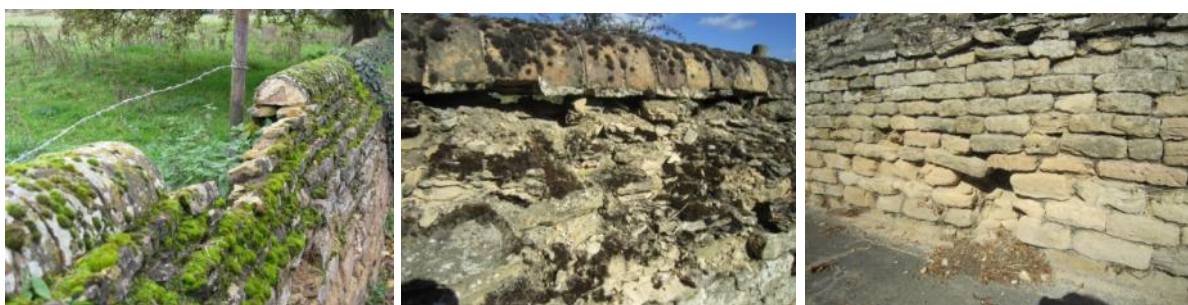
Walls in need of repair
